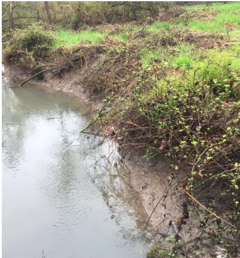
Figure 3.3 Deteriorated areas of bank along the bridge. The GPS coordinates of this area are N45.20316, W123.19923.
